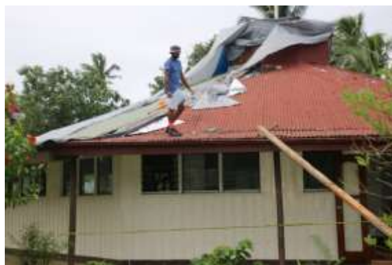
Old chapel normally covered with tarpaulin because of the many leaks
