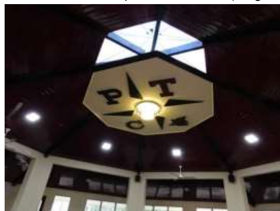
New weatherproof glass ceiling with the PTC logo with new sound system mounted to the walls
